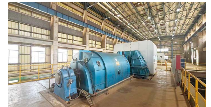
Waste heat recovery equipment
